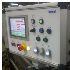
Brand new control interface cabinet with large 8" colour TFT touch-screen interface. Includes push buttons and control label.
