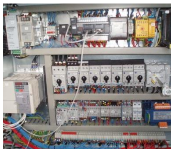
Newly wired cabinet complete with new circuit breakers, contactors, PLC, cutter inverter, safety relay and motor looms.
